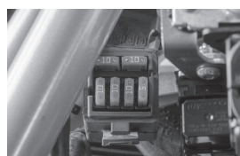
Fuse Box with Cover Open
